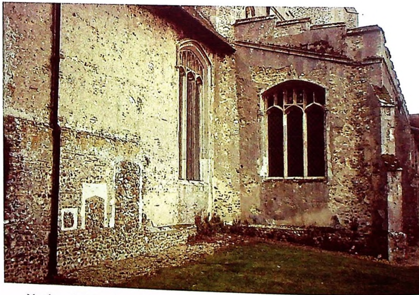
North wall of the chancel, showing the 'scars' of the former chantry chapel. ©
