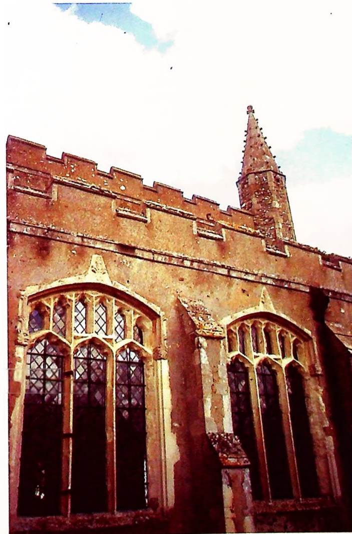
South side of the church, showing hood-mould and dripstones on the aisle windows. ©
