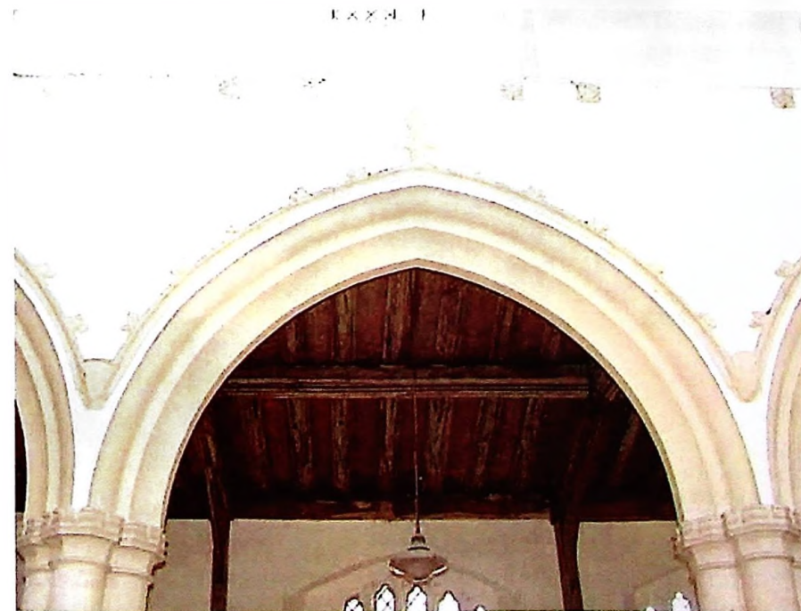
Nave: arcade arch to north aisle. Crocket and finial decoration, with string-course above. ©
