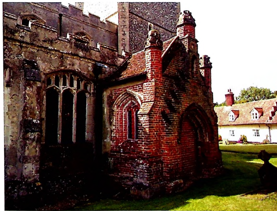
The north porch, built entirely in brick, with a profusion of decorations and mouldings. ©
