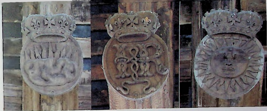
Some of the seventeenth-century royal emblems on the beams of the nave roof
